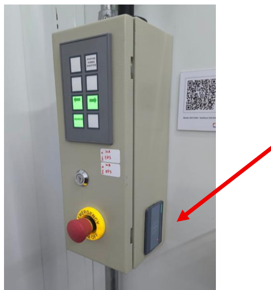
Figure 10: Reader installed on the beamline
