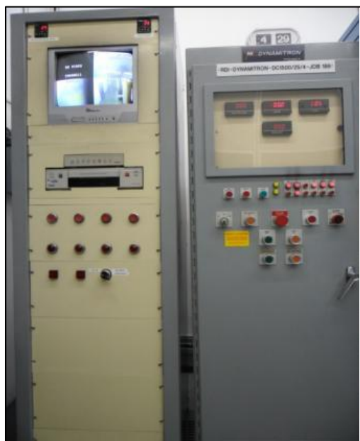
FIG.3: Electron beam control panel.
