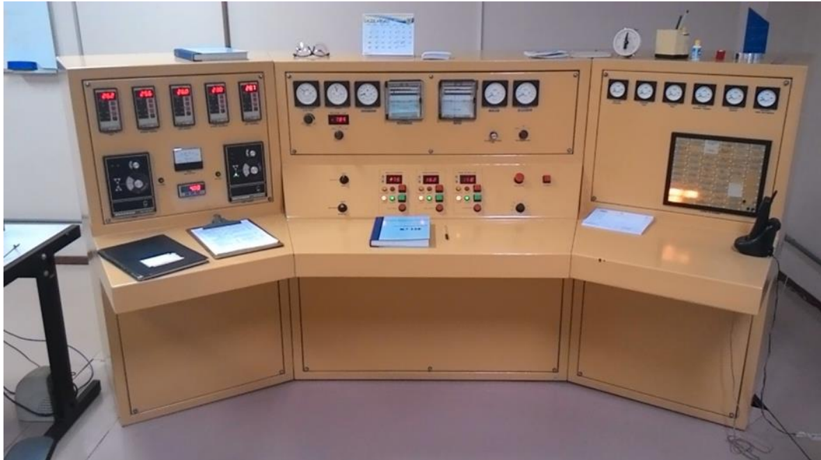
Figure 2: Control panel for the IPR-R1 Triga reactor.
