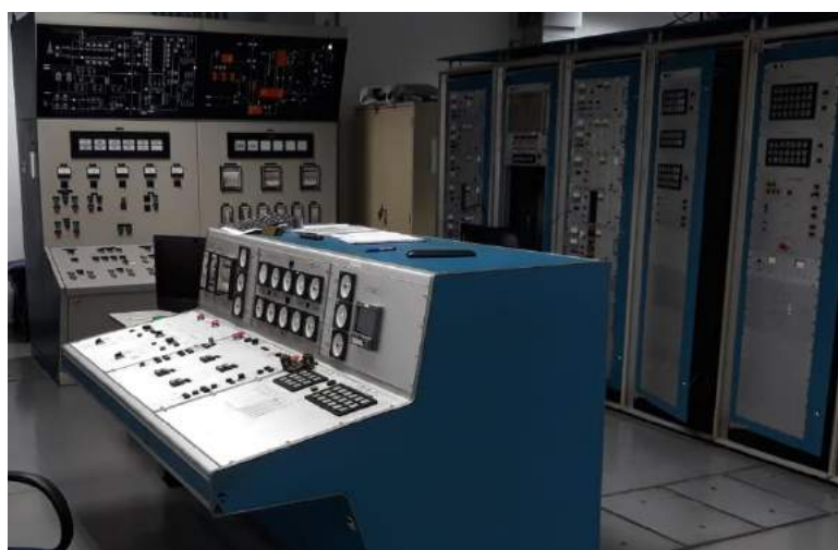
Figure 1: Control room of the Nuclear Research Reactor IPEN/MB-01.
